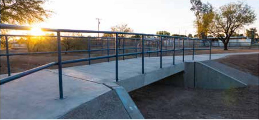
Students at Changemaker High School led the effort to build a new footbridge and sidewalks in the Naylor Neighborhood, paid for by Pima County Neighborhood Reinvestment bonds. The improvements allow people to cross a stretch of road that floods whenever it rains.
