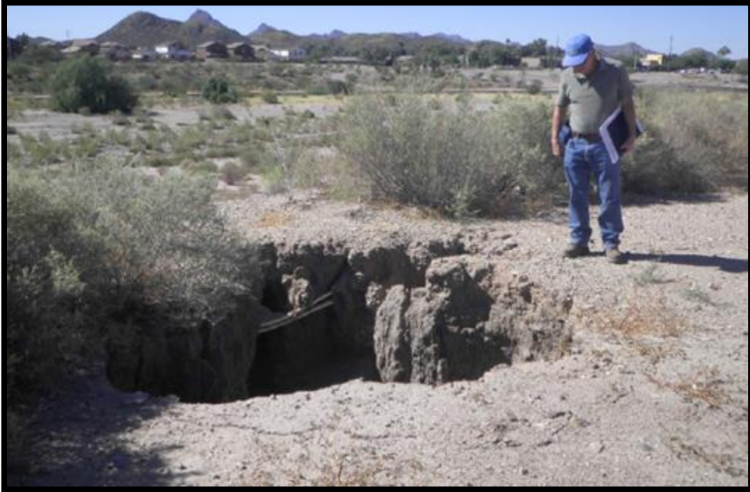
Erosion area within the existing project area. An example of why the City of Tucson has closed this park.
