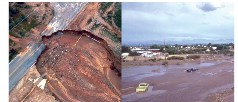
How would you know the pavement was gone if this road were covered with flowing water? At some point, saturated ground gives way and the pavement above it fails...often from the weight of a car. Don't put yourself, your passengers or rescue personnel in harm's way.
