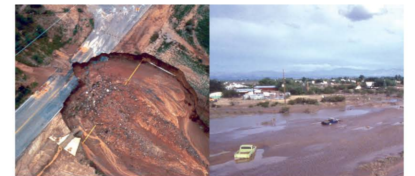
How would you know the pavement was gone if this road were covered with flowing water? At some point, saturated ground gives way and the pavement above it fails...often from the weight of a car. Don't put yourself, your passengers or rescue personnel in harm's way.
