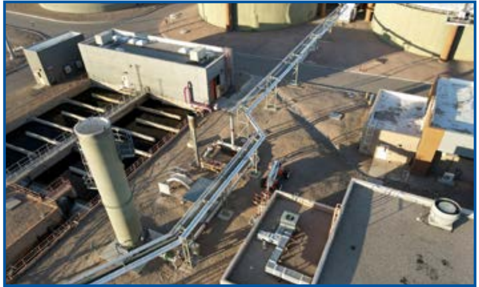
Aerial photo of the biogas pipeline from the digesters to the gas cleaning facility.
